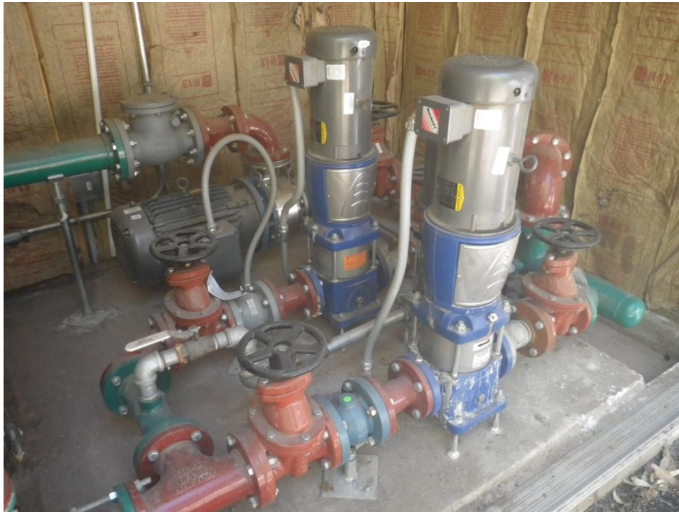
Figure 3. Cramped interior of the Booster Pump Station shed.
